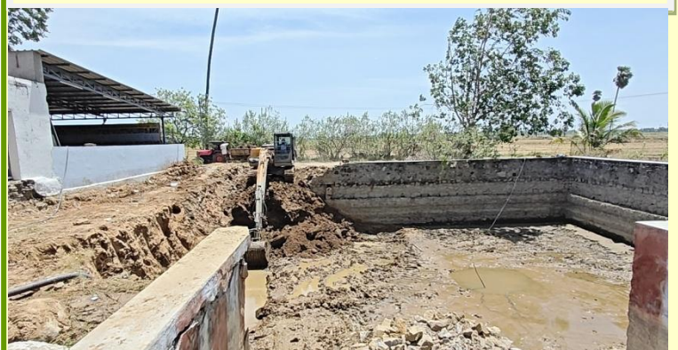
Broken wall because of poor foundation
