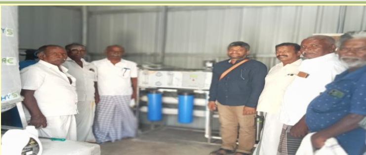
Inspecting the working of the RO plant
