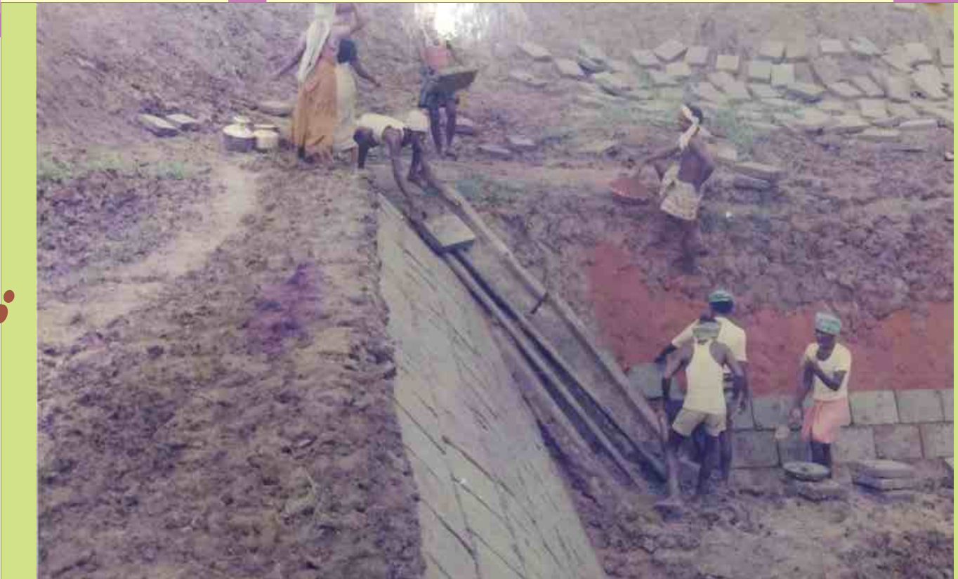
A novel method of pitching the slopes with stones to avoid sliding of the soil
