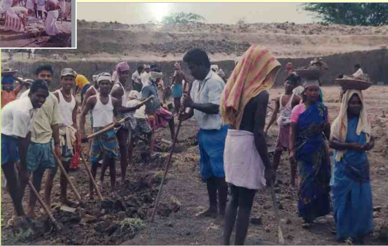
De-silted soil given to the Farmers as a fertilizer in their fields
