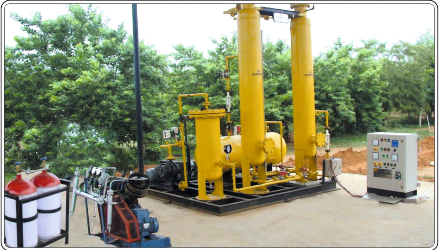
Vacuum pressure swing Absorption (VPSA) system with 2 stage compressor, control panel and CBG cylinders -
