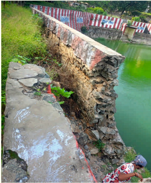
A view of fallen wall
