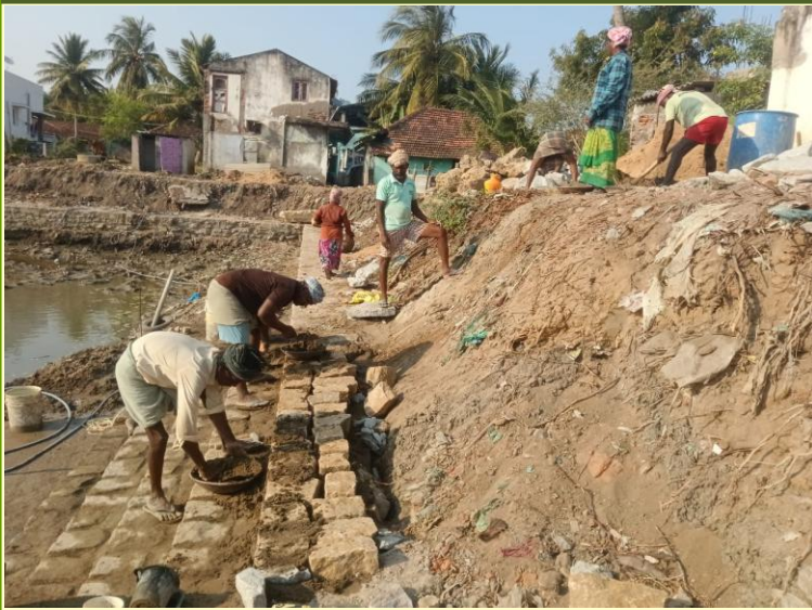
Work of Construction of steps on one side of the entrance is on ..
