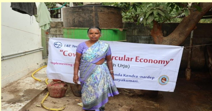
Smt.Murugesan, Perumalpuram posing for photograph with her Bio-methanation plant
