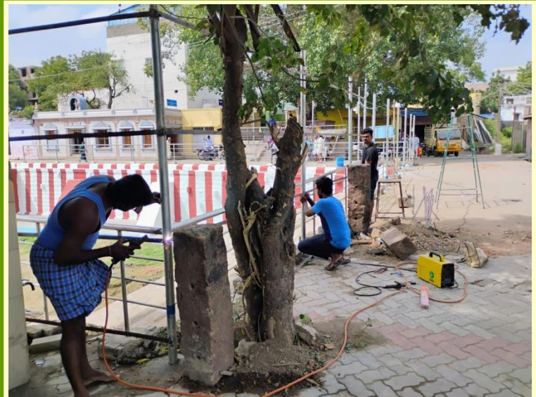
Welding of pipeline is on ..... for providing a jali to protect the Teertham from public throwing the garbage
