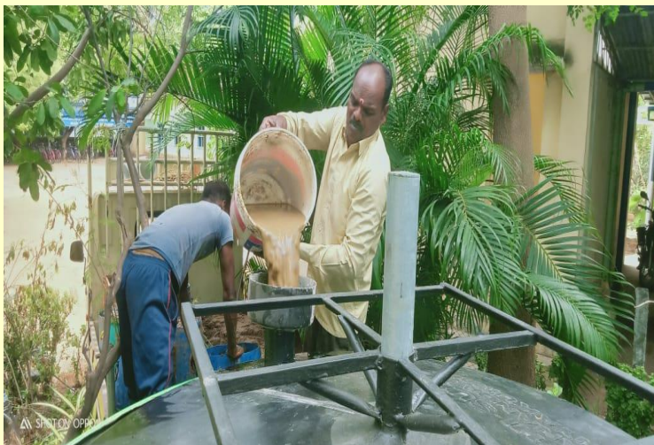
Pouring cow dung slurry to the plant for bacterial colony formation at Govt. Middle school, Alanvillai
